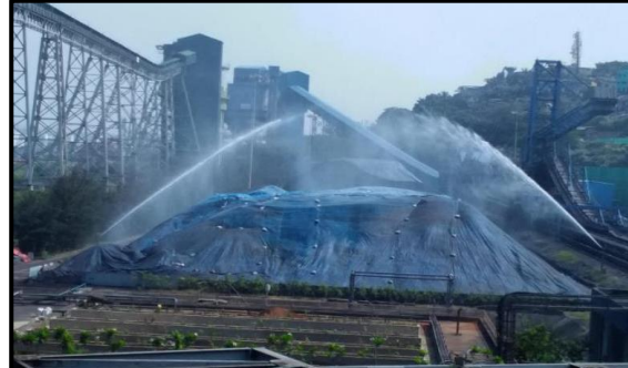
360 deg. Yard Sprinkling System (DSS)
